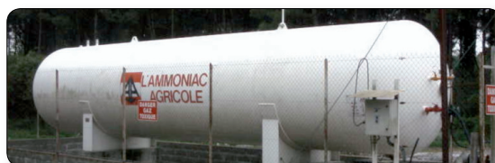
Cuve Ammoniac agricole
